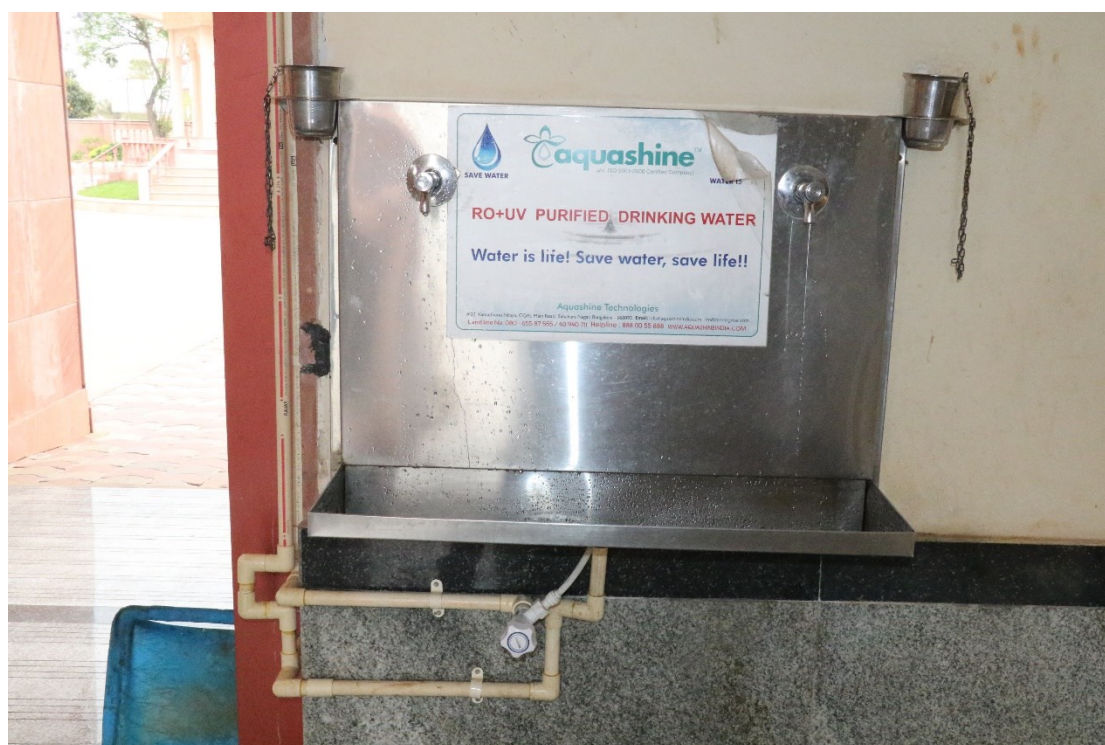
RO water filtration system
