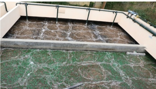
MBBR unit in Sewage Treatment Plant.
