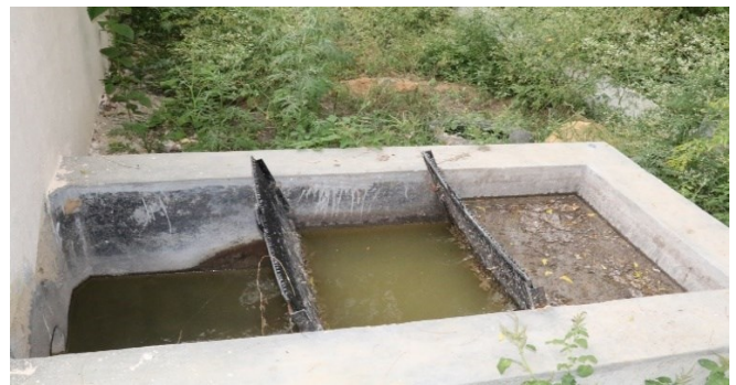
Screening unit in Sewage Treatment Plant.
