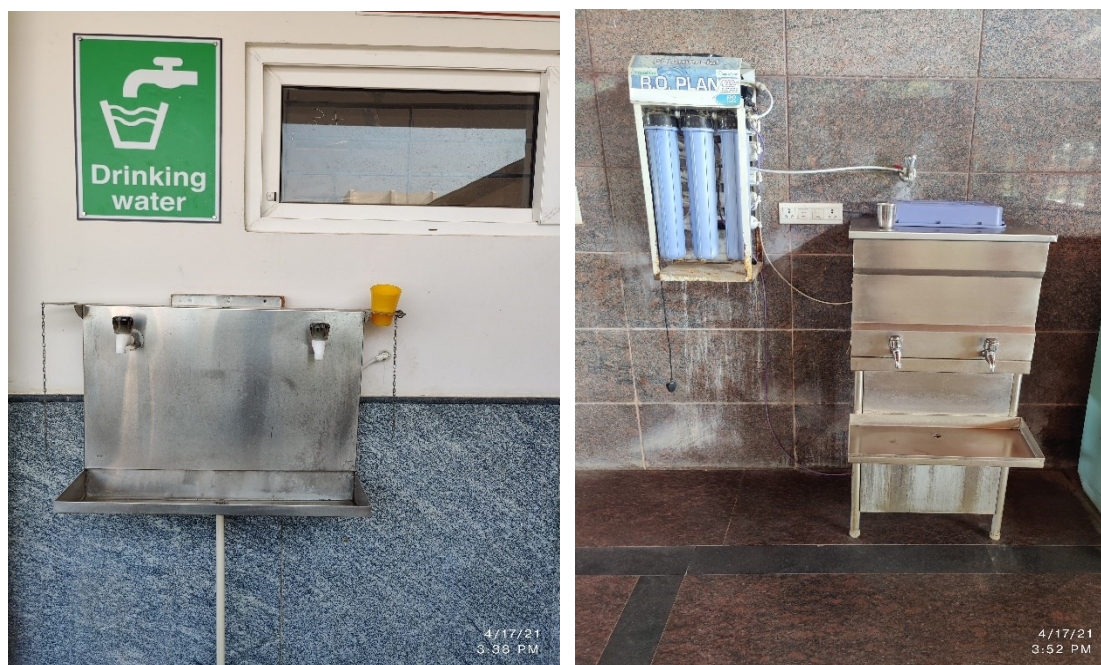
RO water filtration system
