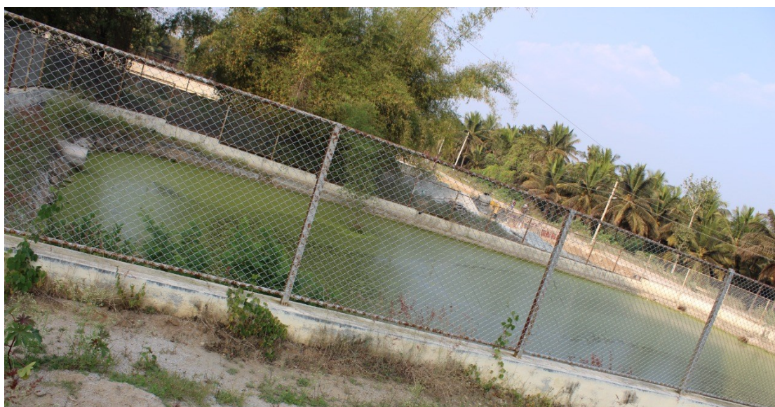
Rain water collection tank
