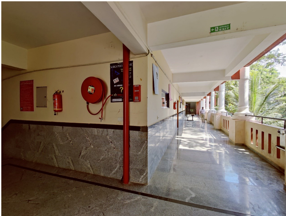
Fire suppression system
