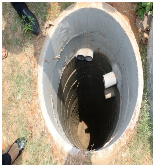
Rain water Recharge Pit
