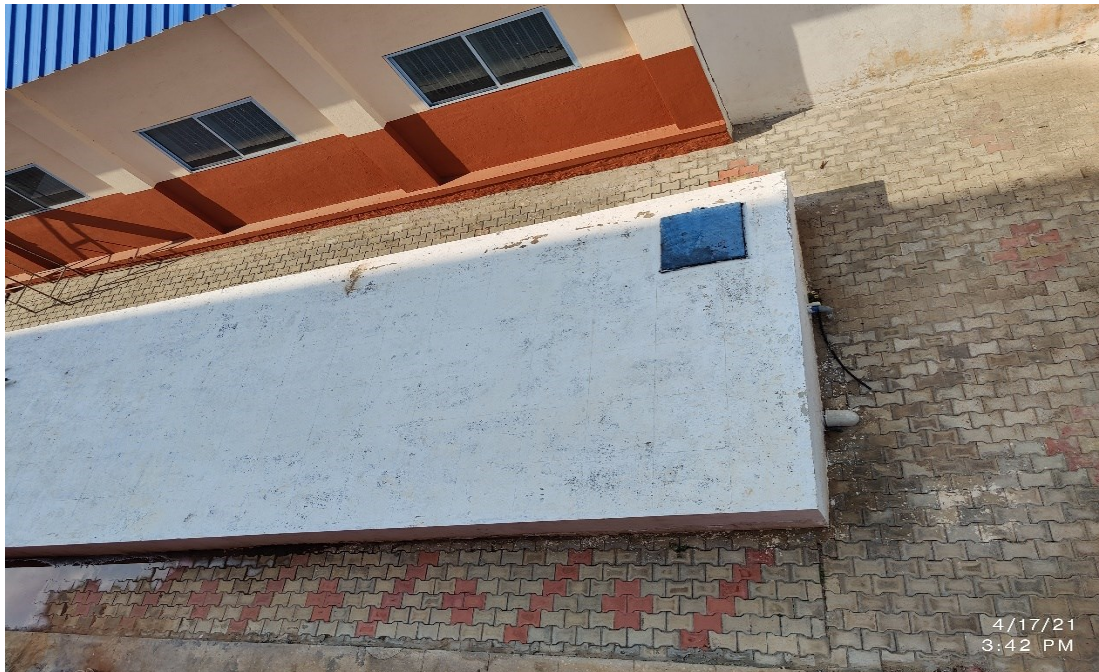
Rain water harvesting tank
