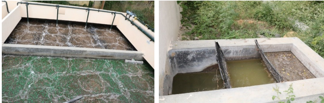
MBBR unit in Sewage Treatment Plant. Screening unit in Sewage Treatment Plant.
