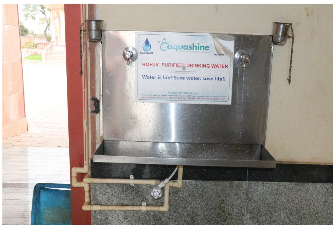
RO water filtration system
