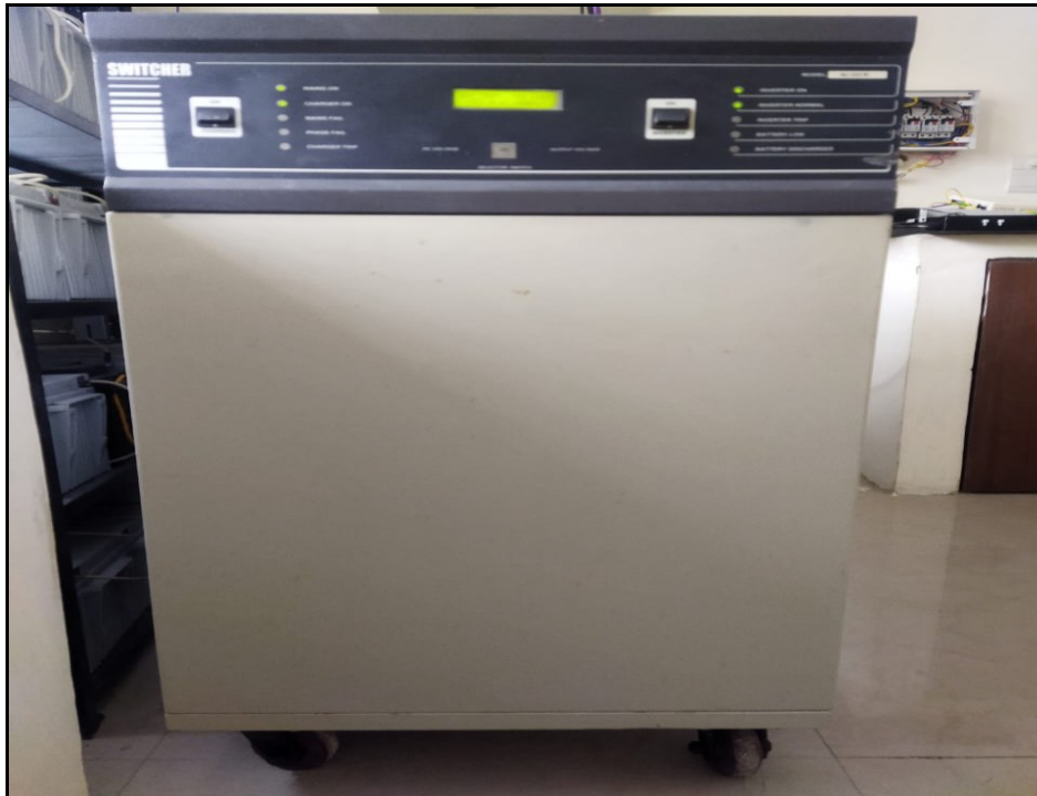
Figure: - UPS System for Emergency Power failure
