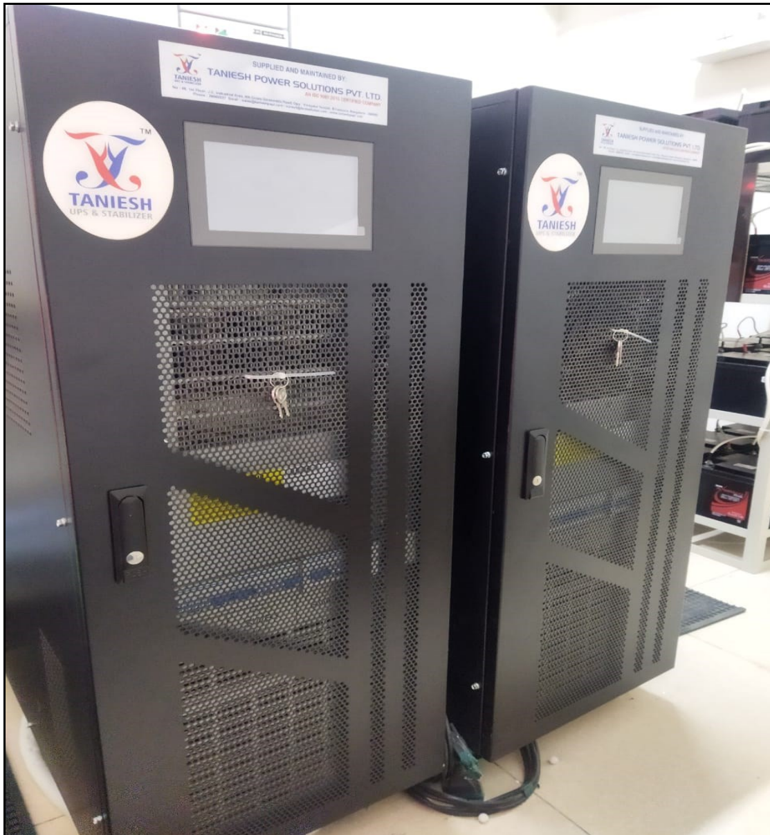
Figure: - UPS System for Emergency Power failure
