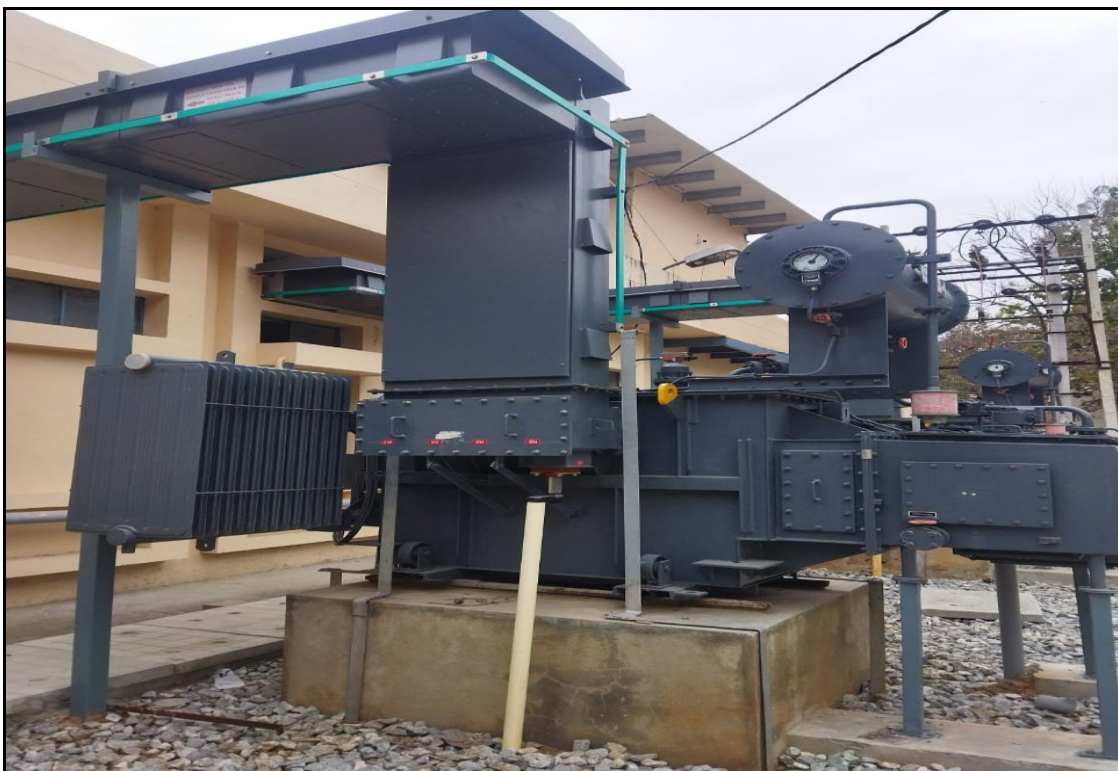
Figure: - 1000 KVA Transformer Photographs
