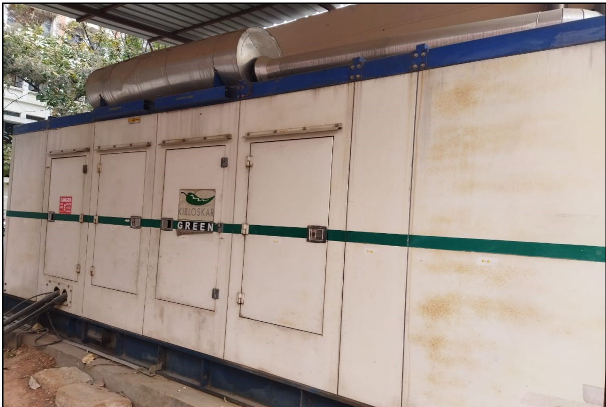
Figure: - DG sets photographs in university
