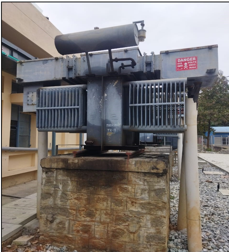
Figure: - 250 KVA Transformer photographs
