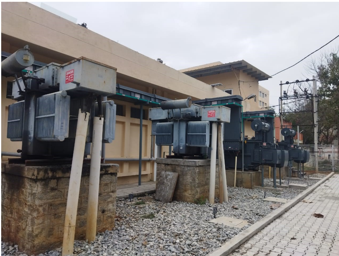
Figure: - 1000 KVA Transformer Photographs
