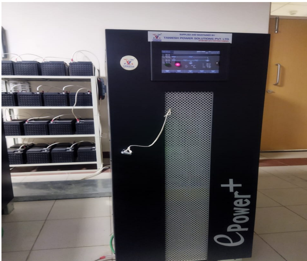
Figure: - UPS System for Emergency Power failure
