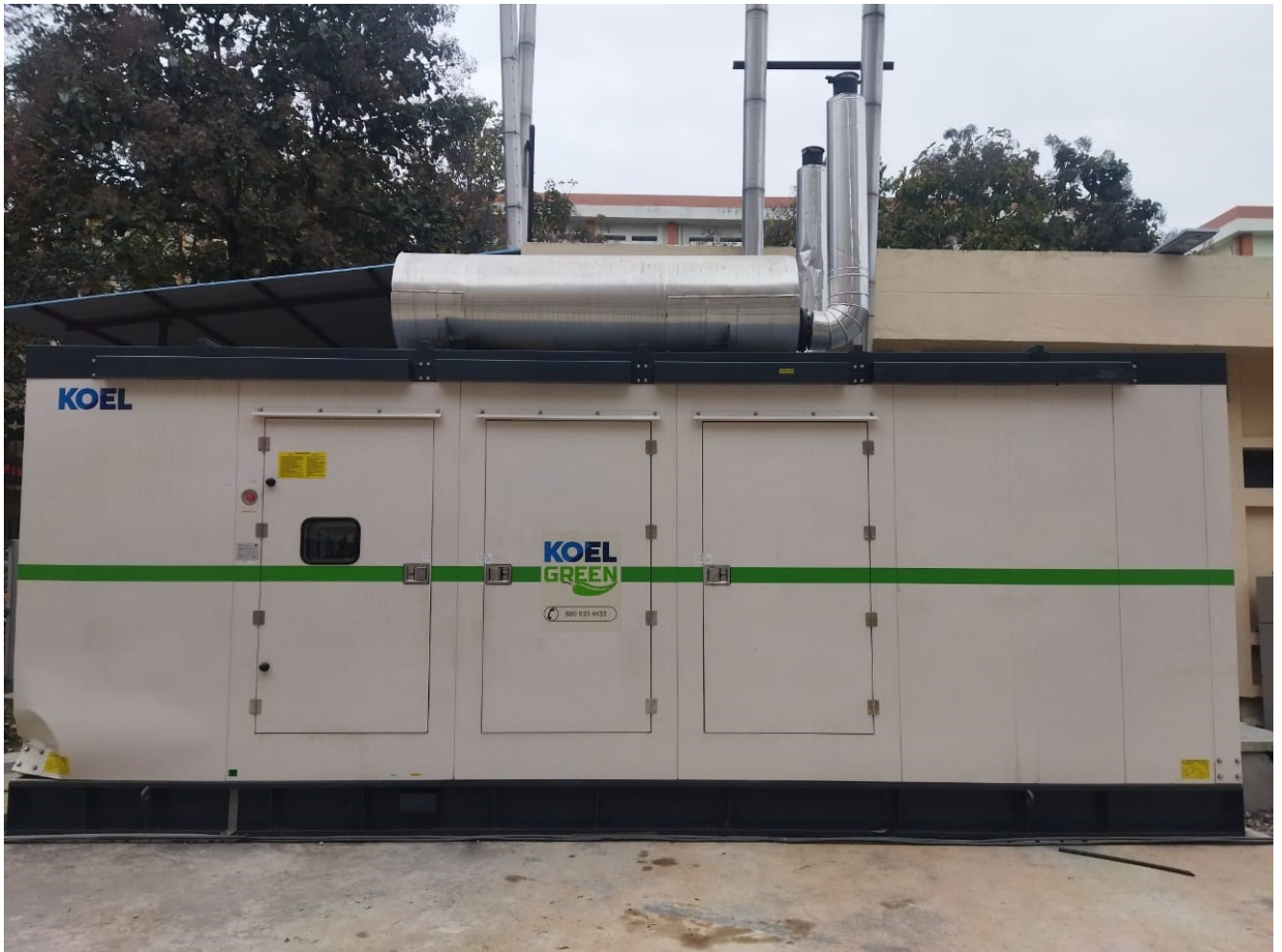
Figure: - DG sets photographs in university
