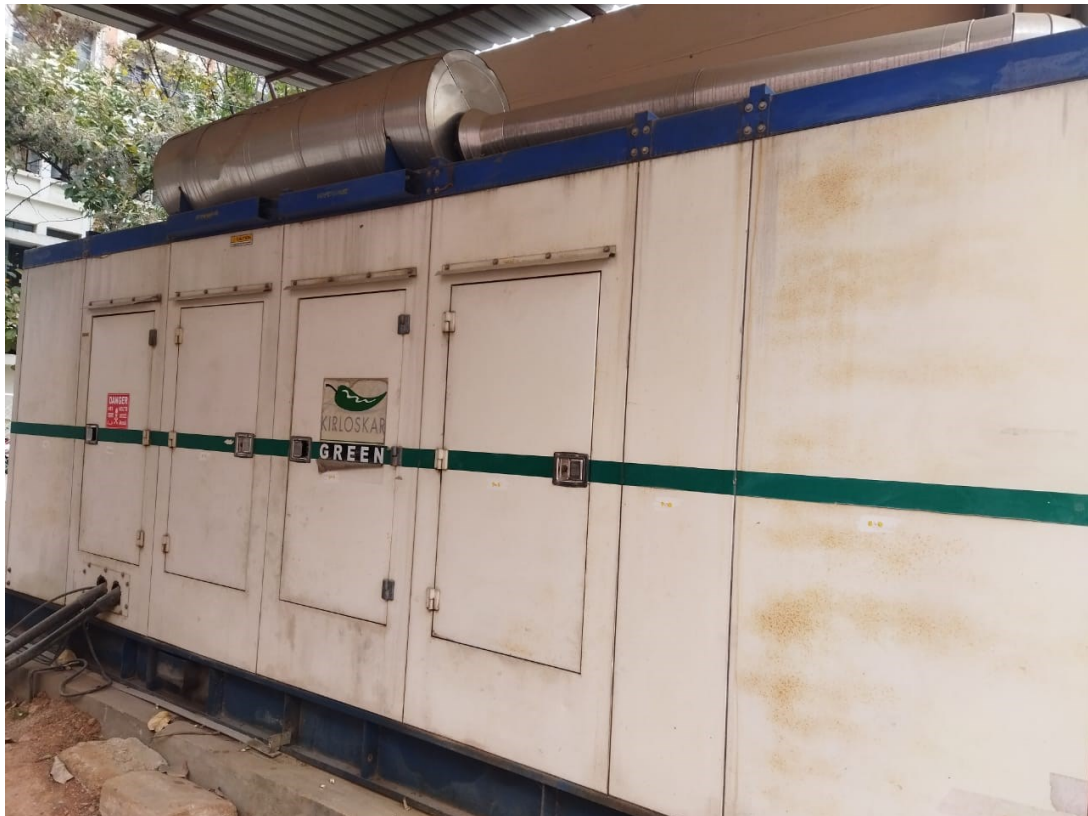
Figure: - DG sets photographs in university
