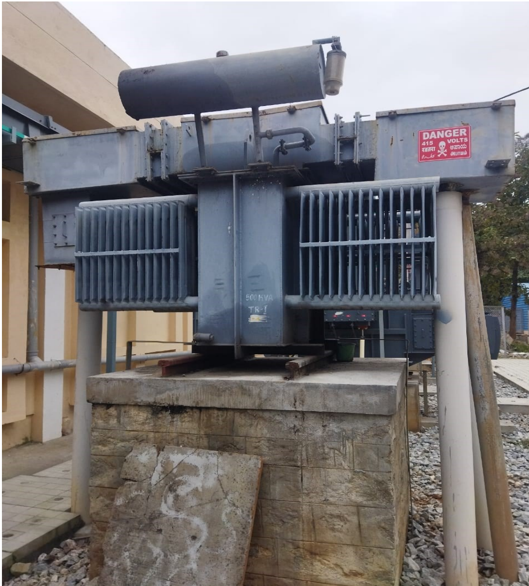
Figure: - Transformer Photographs
