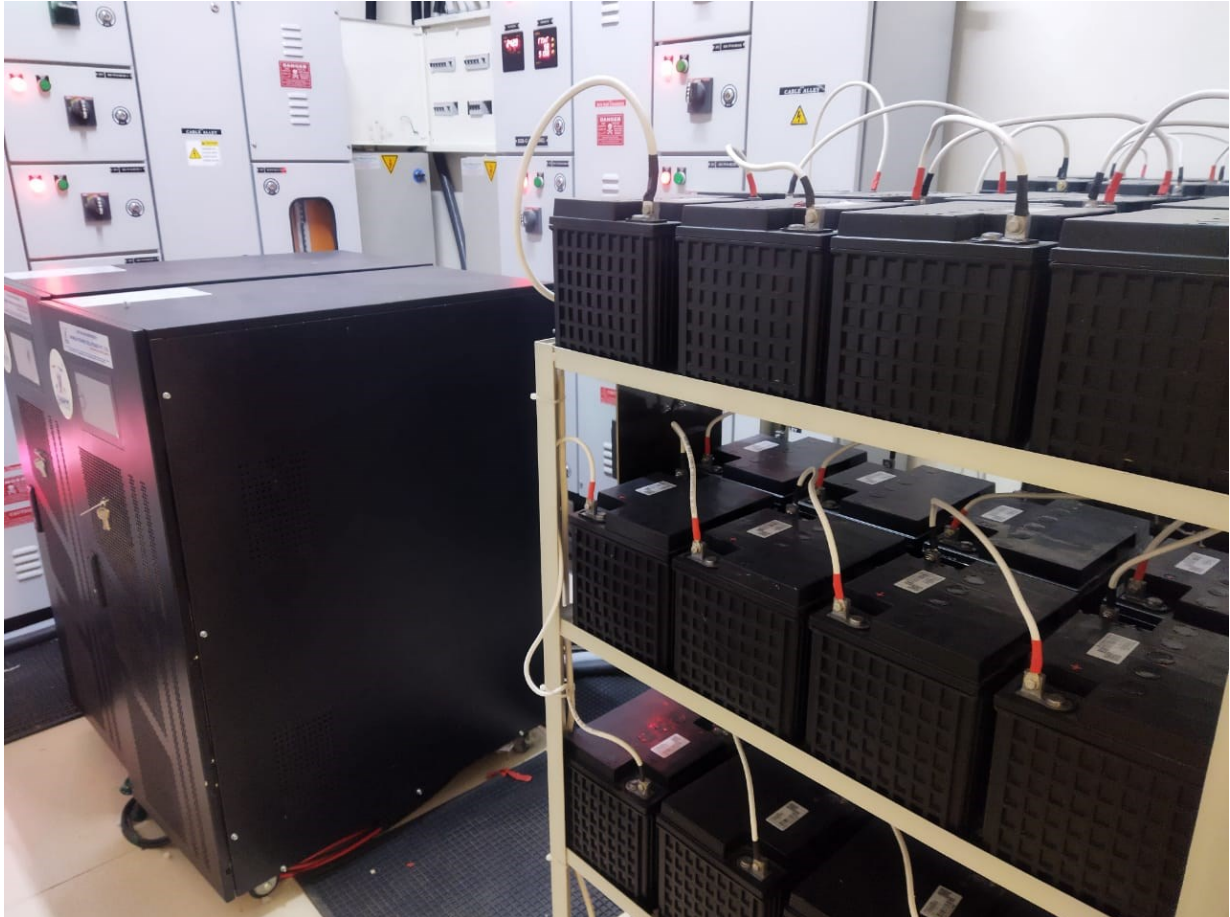
Figure :- UPS System for Emergency Power failure
