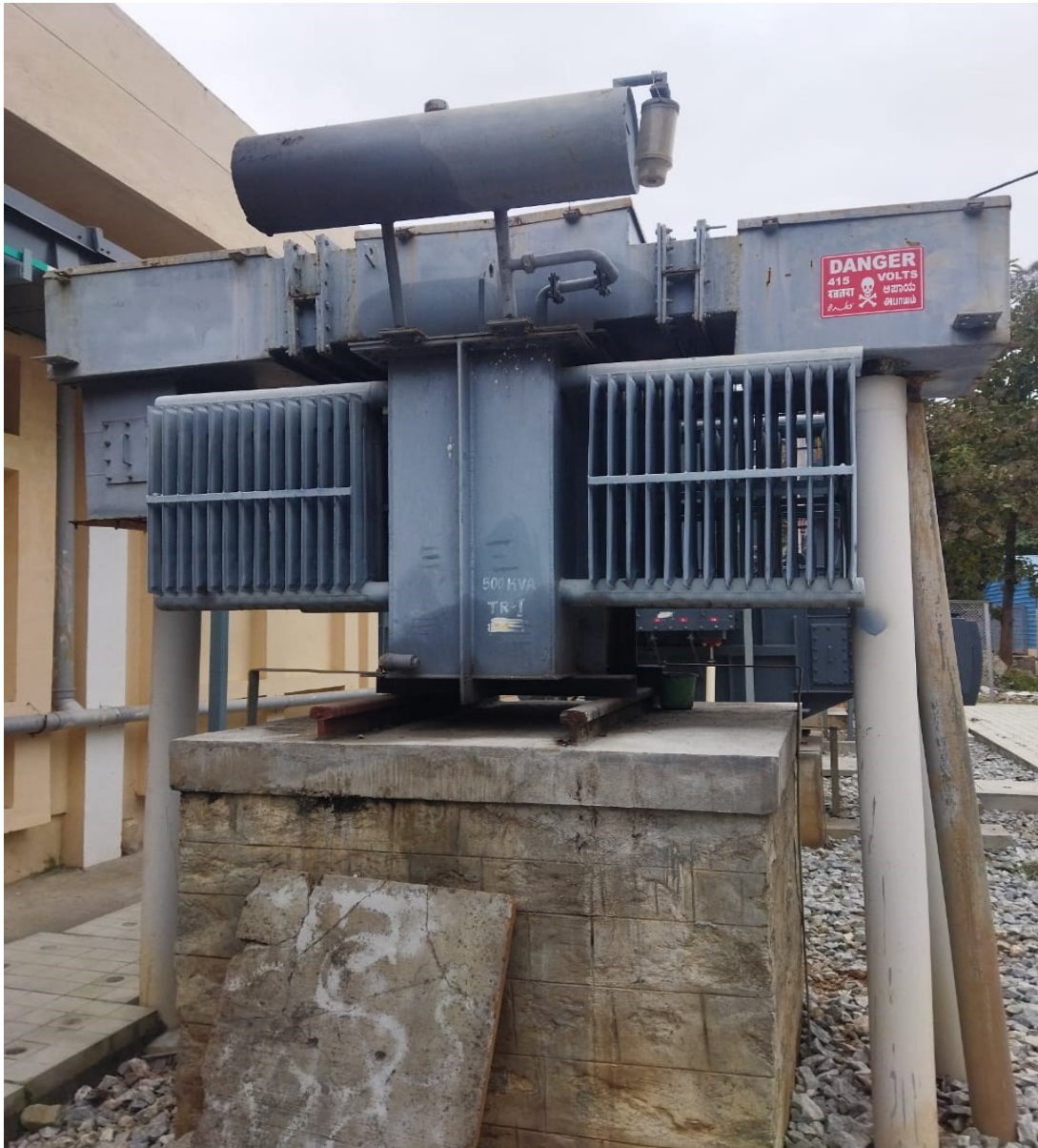
Figure :- 250 KVA Transformer Photographs
